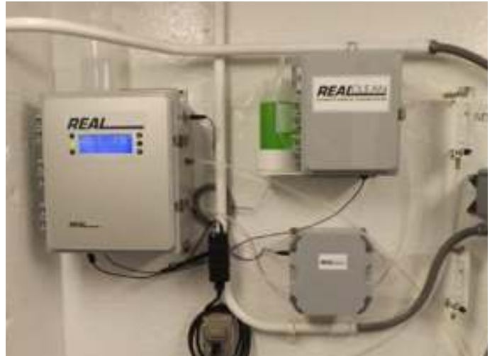
Figure 1: Ridgway WTP's Real UV254 analyzer measuring both raw and finished water with the dual feed system.
